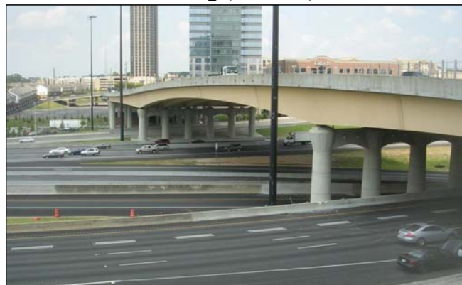
Source: 17 th Street Bridge Canopy Failure Investigation, WJE Associates
